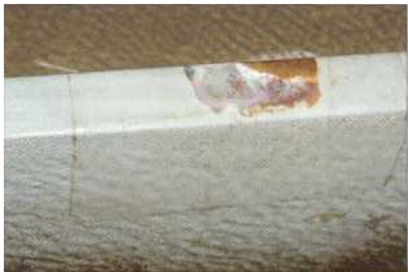
Figures 1 and 2: (at left) show clear fluoropolymer film patches over areas of coating breakdown in a ballast tank of an oil tanker following six months of immersion service. The dark lines in the photos reveal the boundaries of the patches in each picture. Photos courtesy of Integument Technologies, Inc.
